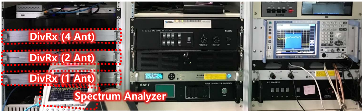
<Measurement Facility with Diversity Rx Sets>
