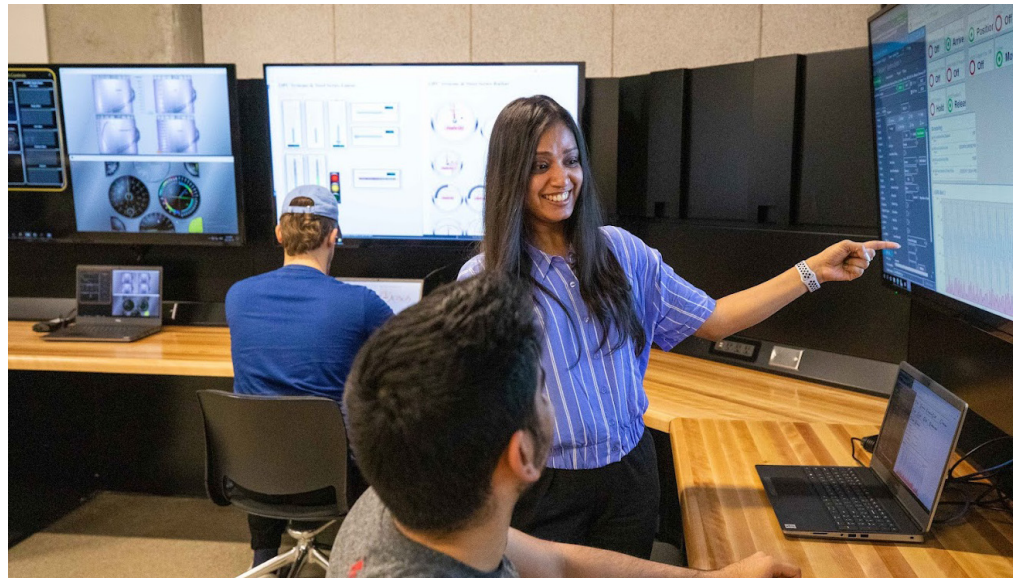
Pictured above (L-R): Alex Mosor, student; Hartej Tapia, student; and Pallavi Gupta, project coordinator collaborate on performative maintenance initiatives from the Cisco Digital Transformation Zone data centre in the Barrett CTI. This data centre is capable of monitoring Internet of Things (IoT) smart devices and systems within the building.
